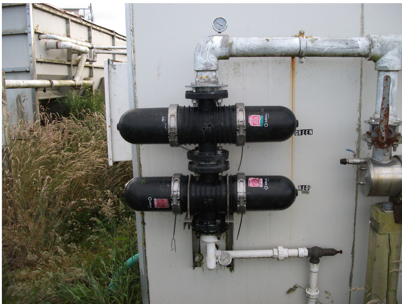
Waste Water Filters Prior To UV Treatment And Onto Irrigation Fields
