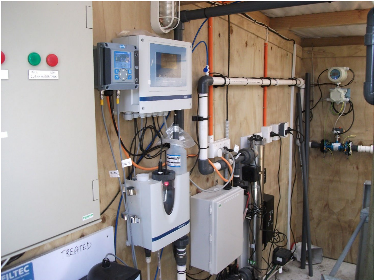
Kaingaroa Water Plant Control Panels
