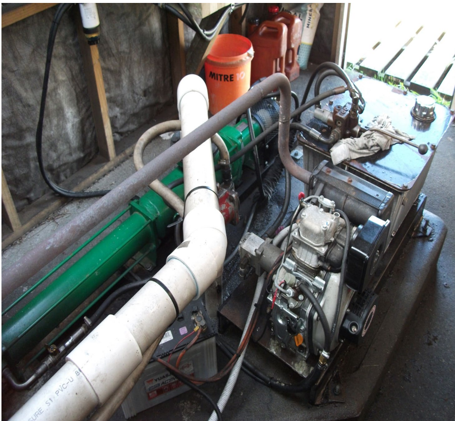
Lake Rangitai Raw Water Pump & Motor
