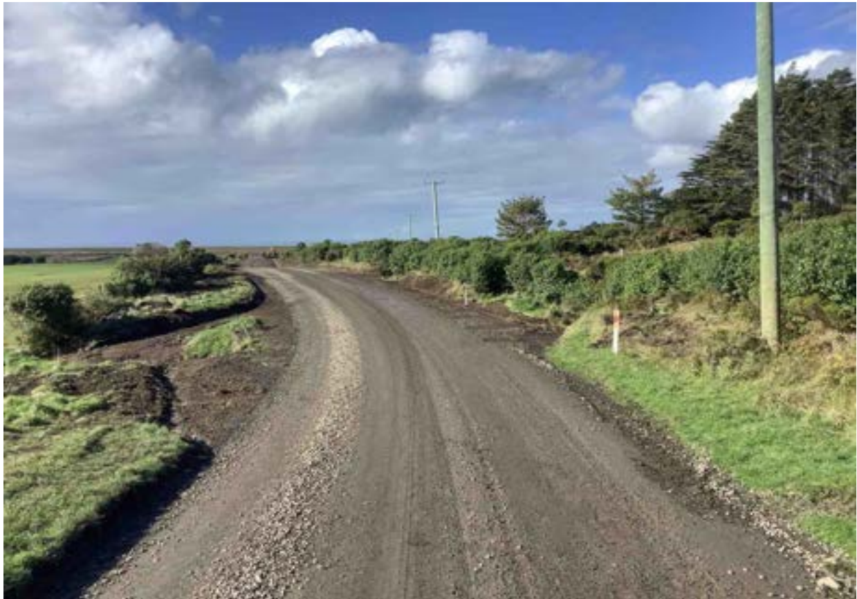
Watertabling On WW-O Road
