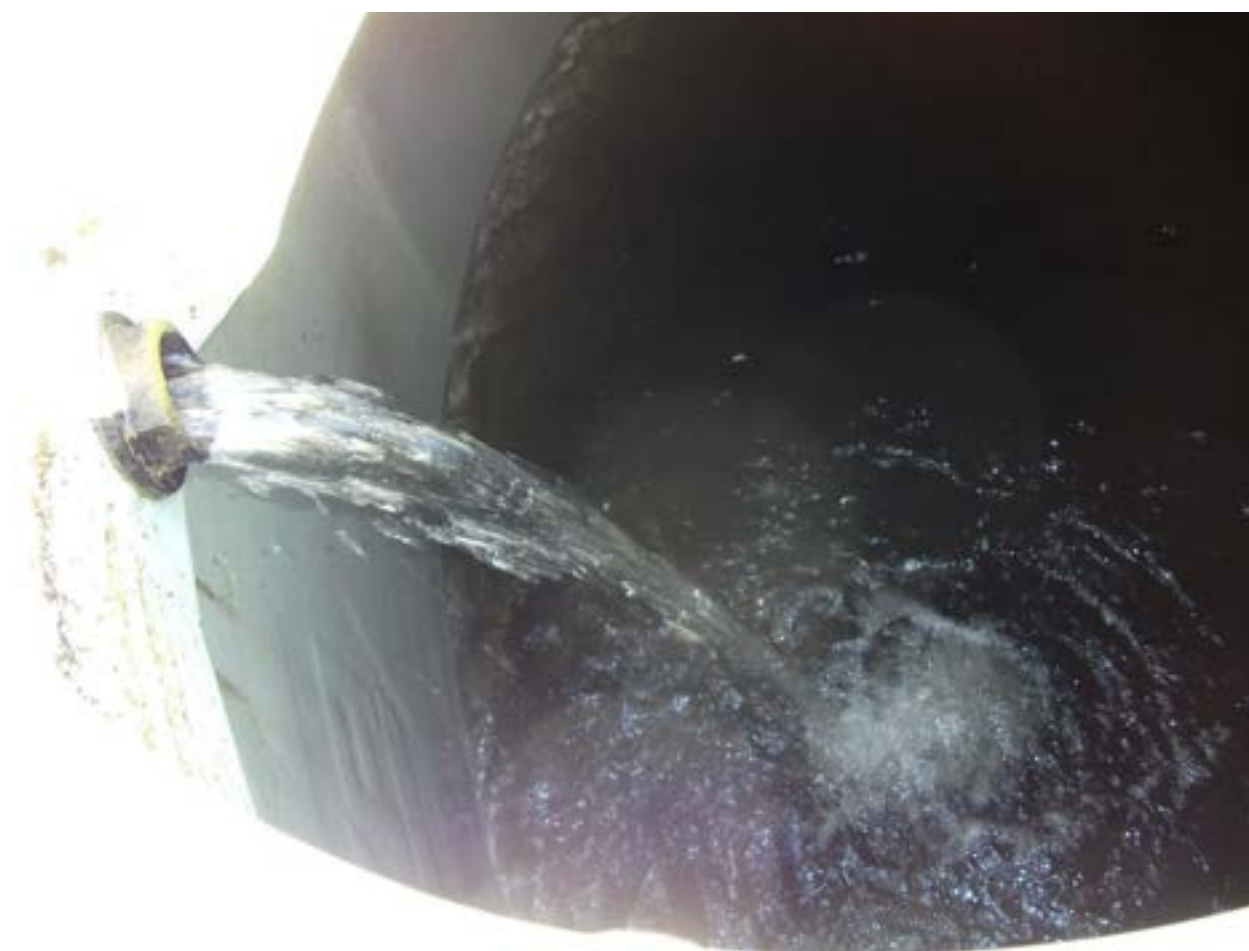
Raw Water From Lake Rangitai Entering Storage Tank At The Kaingaroa Water Plant
