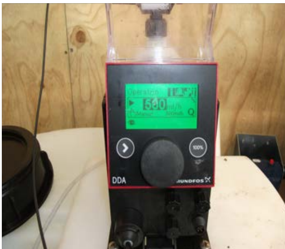
Kaingaroa Water Plant Chlorine Dosing Pump
