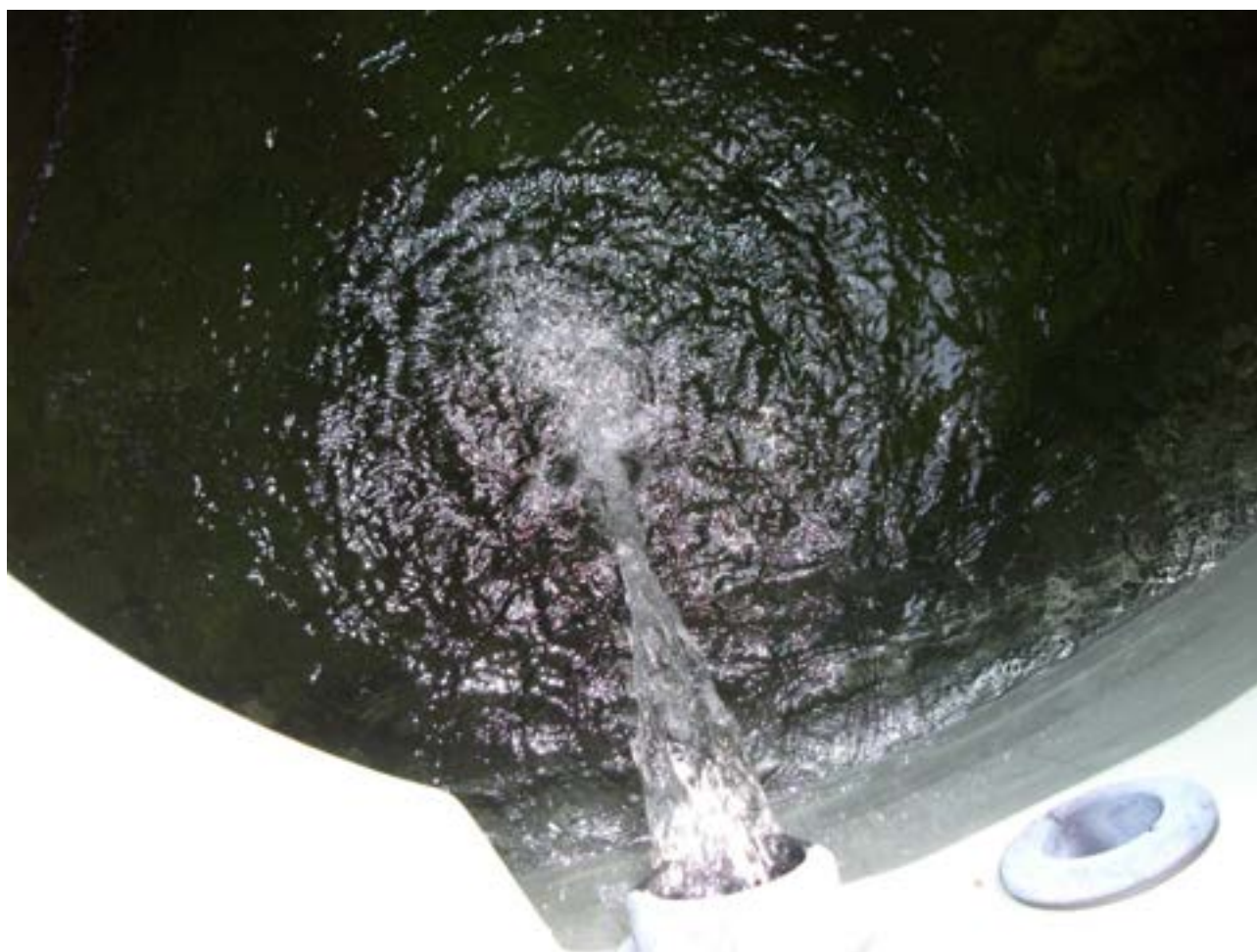
Treated Water Entering Storage Tank At Kaingaroa
