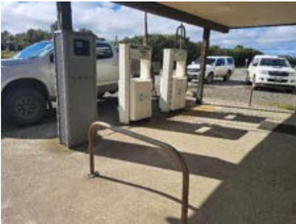
Fig. 69: Fuel spills evident on forecourt, both historic and recent. No bunding to prevent discharge to permeable area.
