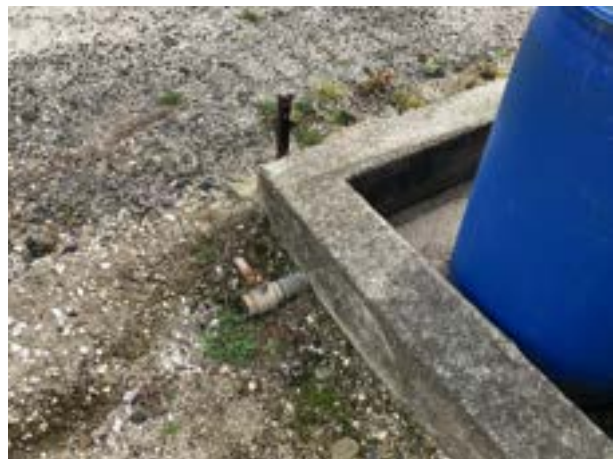
Fig. 29: Stormwater valve left open in bund.
