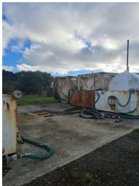
Fig. 64: Fuel tank storage area.
