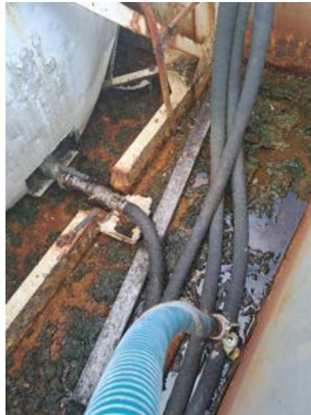
Fig. 68: Inside of bunding on one tank show hydrocarbon sheen and rust.
