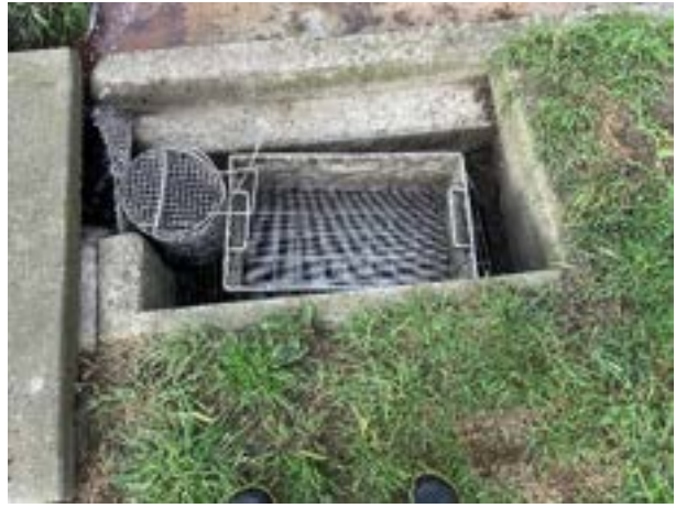
Fig. 15: Solid waste screen into underground storage tank.
