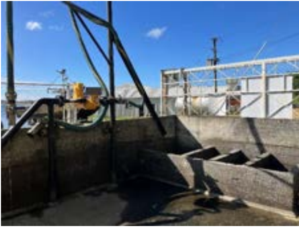
Fig. 73: Spills within bunding.
