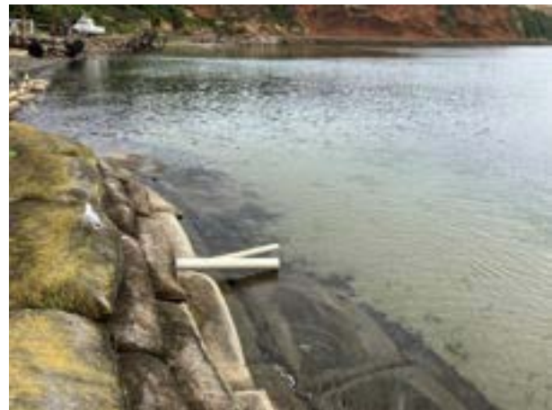
Fig. 10: Discharge pipe to the Coastal Marine Area.
