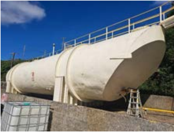
Fig. 71: 400,000L storage tank.
