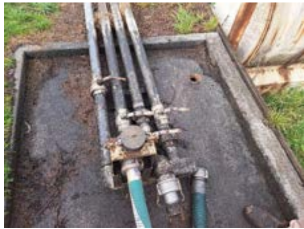
Fig. 4: Leakage of fuel evident on concrete pad.
