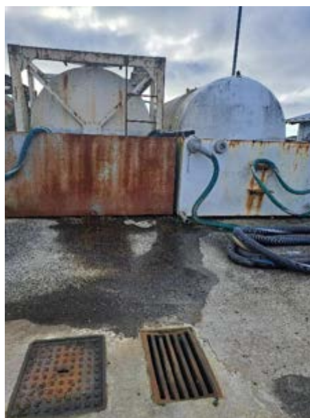
Fig. 66: Stormwater release valves on all bunds were open allowing the discharge of contaminated water.
