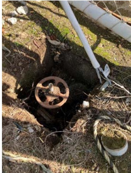
Fig. 74: Release valve left open draining oil to land and CMA.
