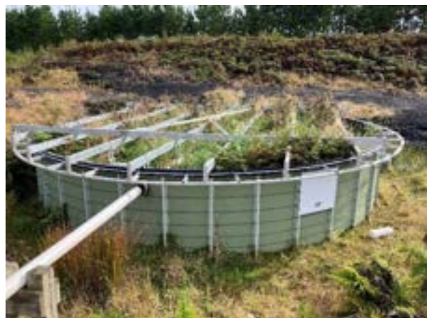
Fig. 100: Overgrown treatment tank.
