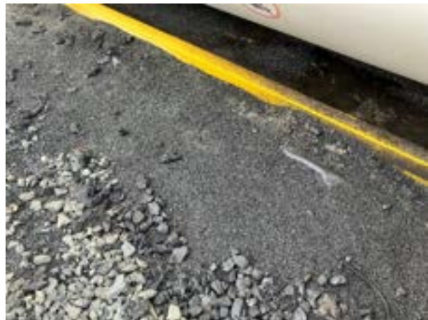
Fig. 27: Sand used to clean up spill left in bund.
