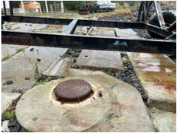
Fig. 82: Disused underground storage tank for trade discharge.
