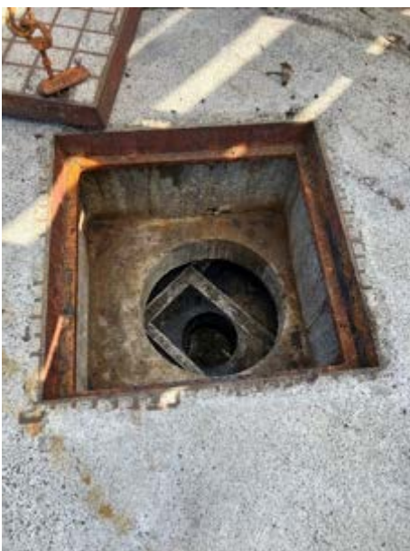
Fig. 79: Underground effluent storage tank.
