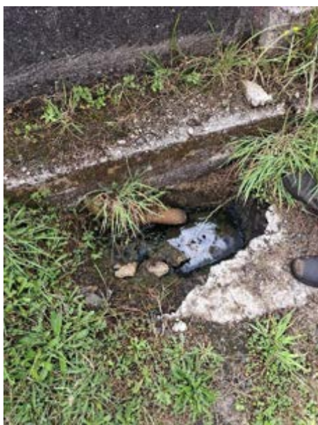
Fig. 1: Open interceptor. Discharge of contaminants to land. Requires clearing and a shut-off valve.
