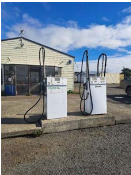
Fig. 63: Fuel bowsers on concrete pad.
