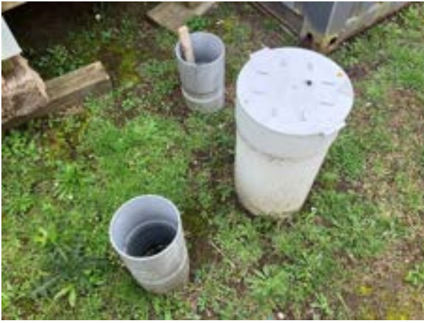
Fig. 14: Underground storage tank off gas pipes.
