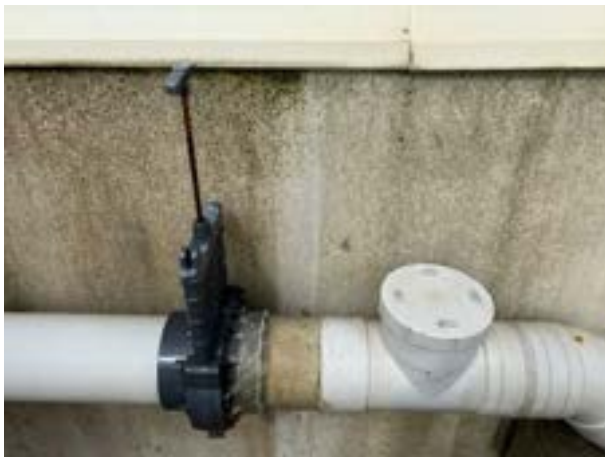
Fig. 9: Shut-off valve on outlet pipe.
