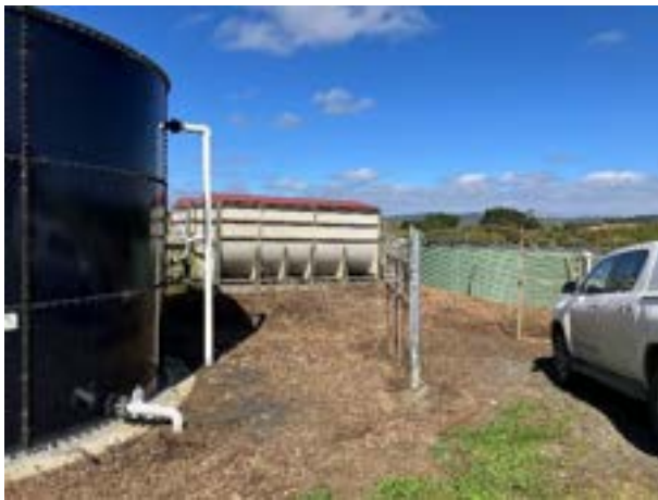
Fig. 91: New settling tank. Perimeter fencing incomplete.
