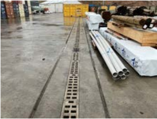
Fig. 81: Stormwater strip drains leading to shut-off valve (then sea).
