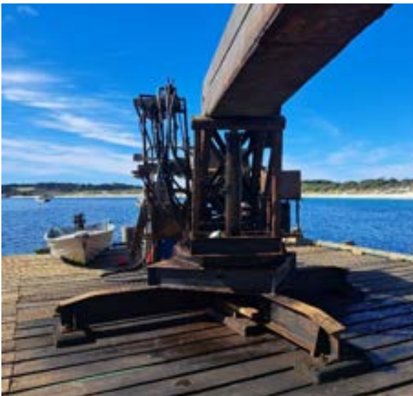
Fig. 87: Crane on wharf leaking lubricating oil and rust onto wharf structure.
