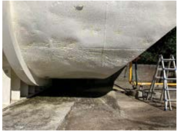
Fig. 72: Walls of the tank compromised.
