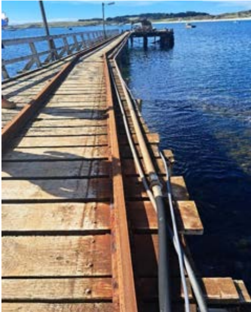
Fig. 85: Wharf structure with new fuel pipeline.
