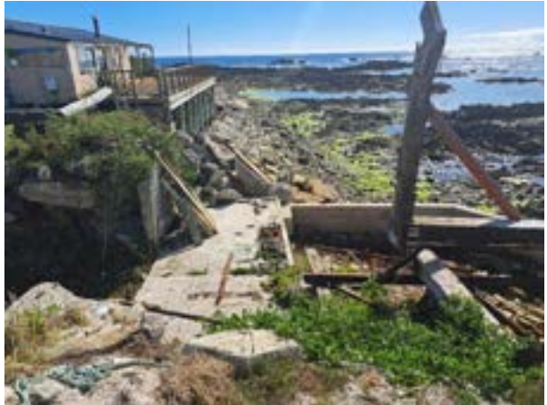
Fig. 86: Coastal erosion at the base of the wharf structure.
