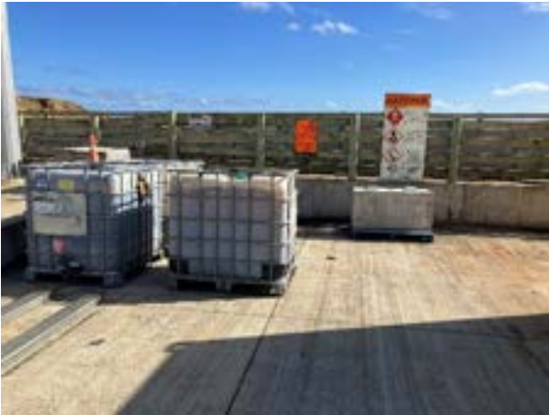
Fig. 75: Hazardous substance storage area (<72 hrs).
