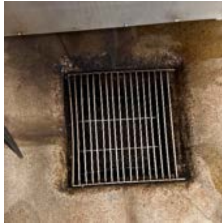
Fig. 17: Solid waste grate under sump in processing room.
