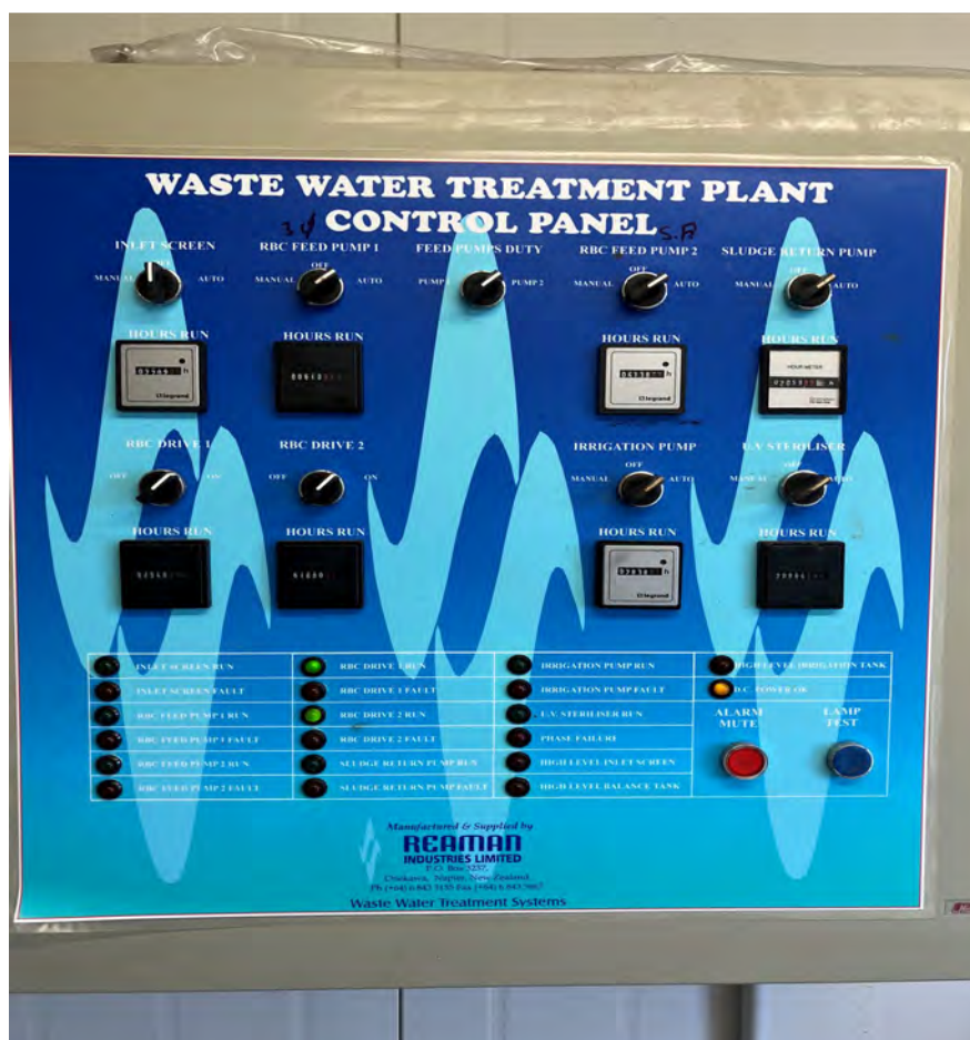
WWWT Plant Control Panel
