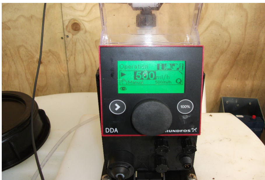
Kaingaroa Chlorine Dosing Pump
