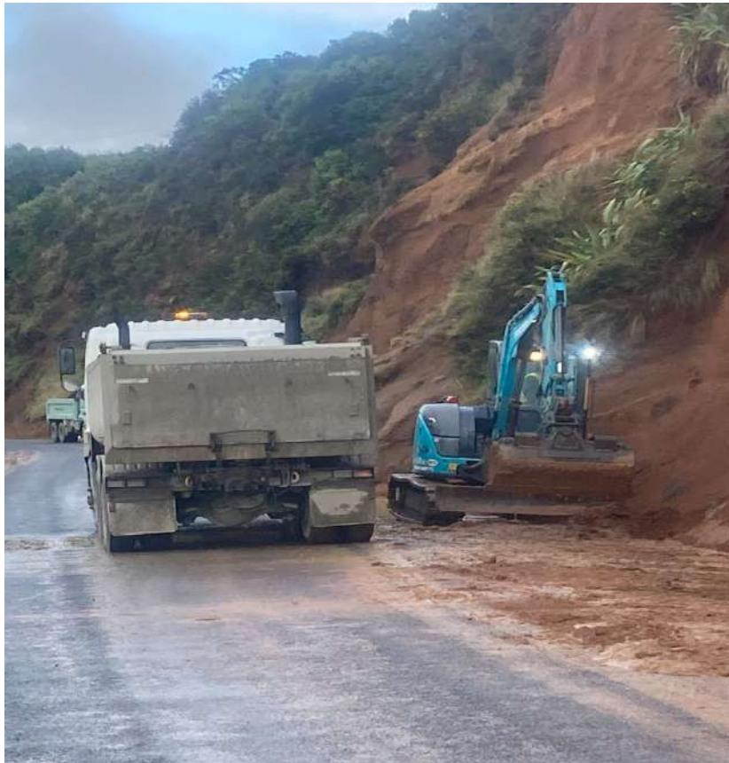
Slip Removal After Heavy Rain Events.
