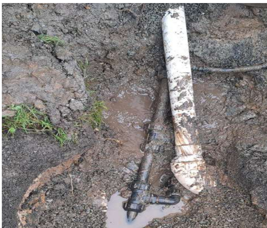
Water Leak At The Council Flats.
