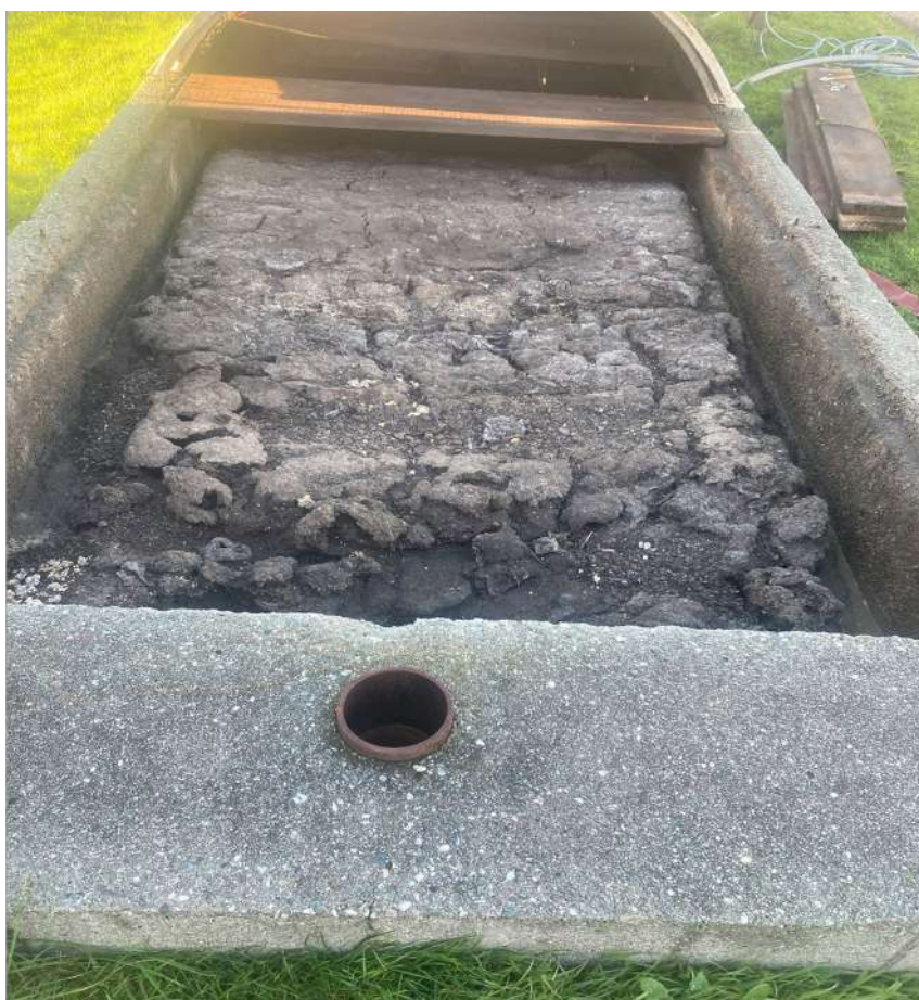
Solids Tank Before Cleaning.
