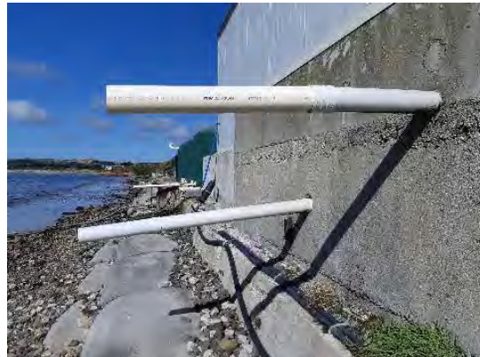
Fig. 9 Discharge pipes to the coastal marine environment
