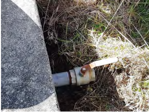
Fig. 32 Stormwater valve on bunding open
