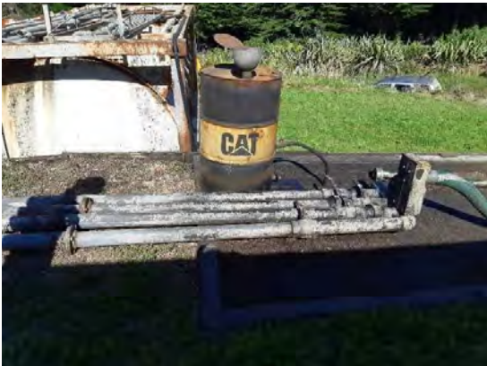
Fig. 4 Leakage of fuel evident beyond concrete pad and wall
