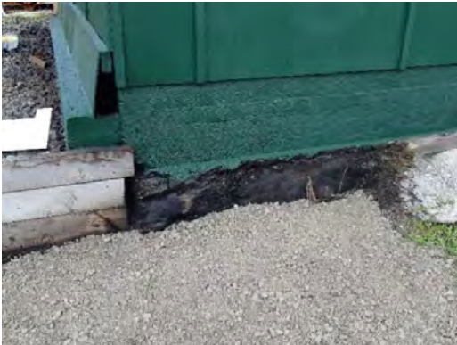
Fig. 15 Leaching of diesel to foundations of diesel generator shed
