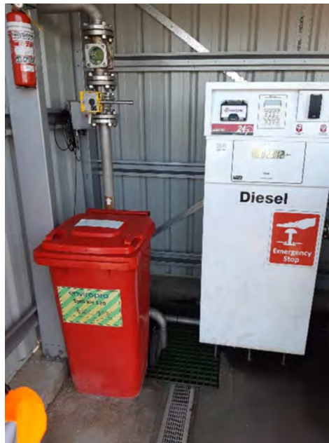
Fig. 73 Pump locked in adjacent shed and spill kit present
