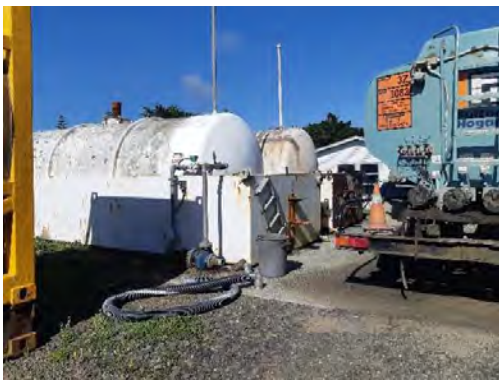
Fig. 67 Bulk fuel storage tanks
