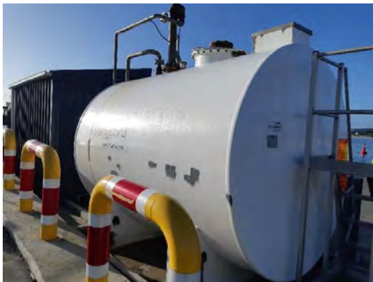
Fig. 72 10,000 litre double skinned diesel tank on wharf
