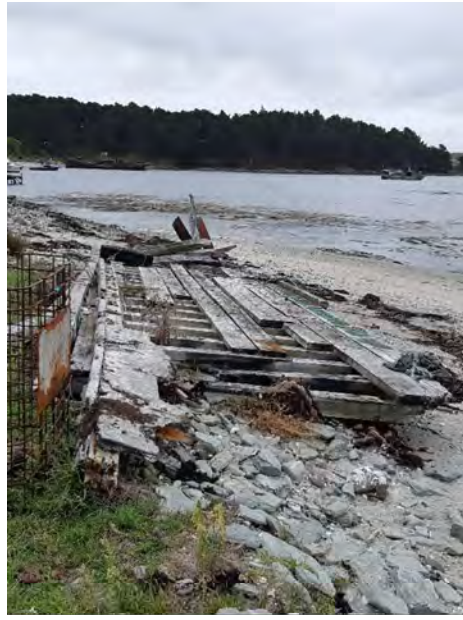
Fig. 90 Section of wharf washed up further down the beach
