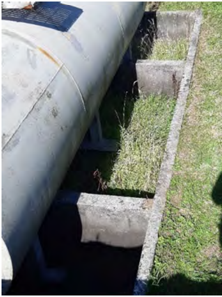
Fig.2 Bunding filled with vegetation
