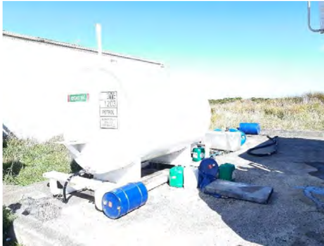
Fig. 29 Bulk fuel storage 5000 litres
