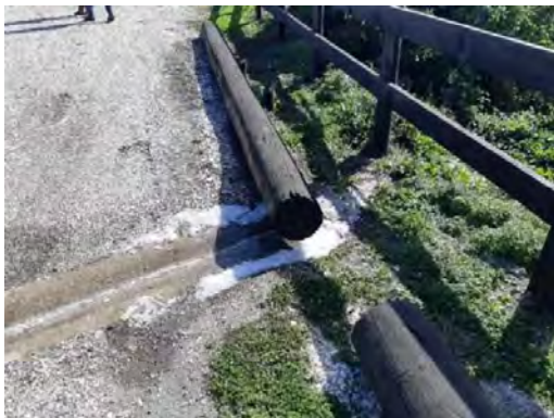
Fig. 22 Factory discharge close up
