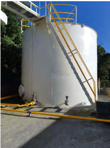
Fig. 83 Bulk storage of diesel
