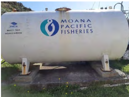
Fig 8. Double skinned diesel fuel storage
