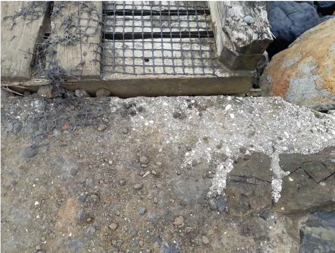
Fig. 92 Erosion of land away from beginning of wharf
