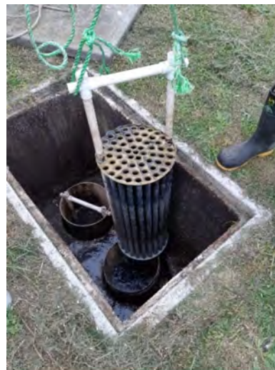
Fig. 18 Factory waste filtering and screening system
