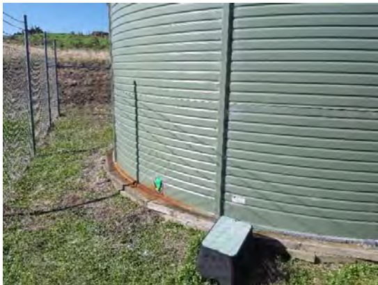
Fig 102. Settling tank with temporarily Fixed hole
