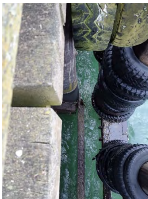
Fig. 94 Erosion of infra-structure of wharf since construction
