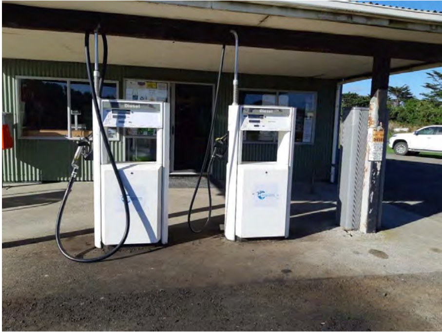
Fig. 71 Fuel spills evident on forecourt
