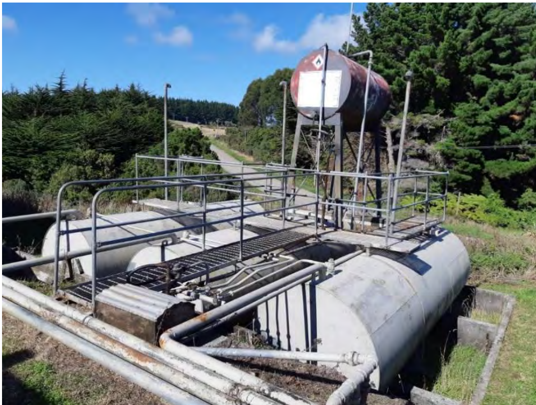
Fig.1 On site Diesel Storage
