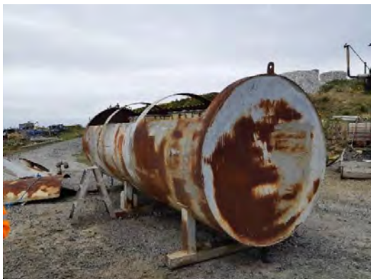
Fig. 10 Makeshift bunding for diesel storage
