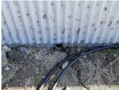
Fig. 23 Discharge pipe for new shed directly to ground.
