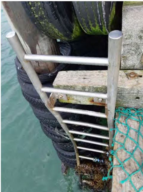
Fig. 93 Illegal ladder attached to wharf
